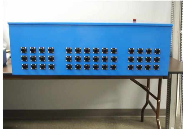
System PLC/Control Enclosure
